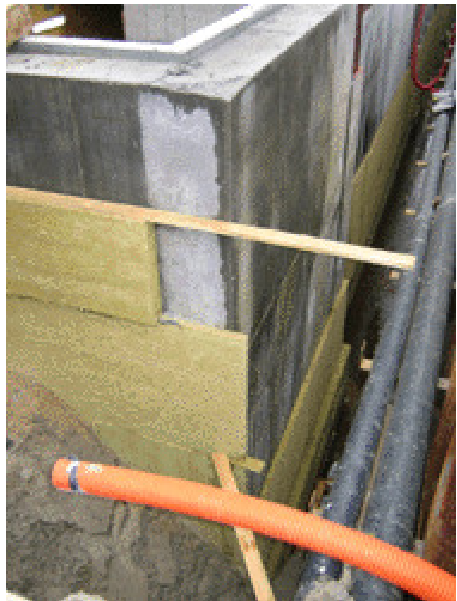
Figure 3: Rock Wool Barrier
